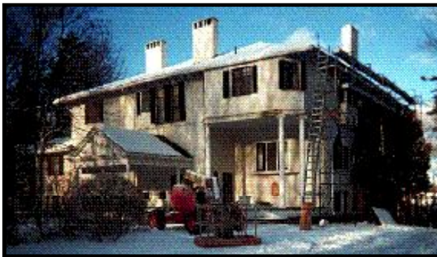
HOPKINS COTTAGE - BAR HARBOR, ME Complete rewiring for restoration of early 1900's summer cottage
